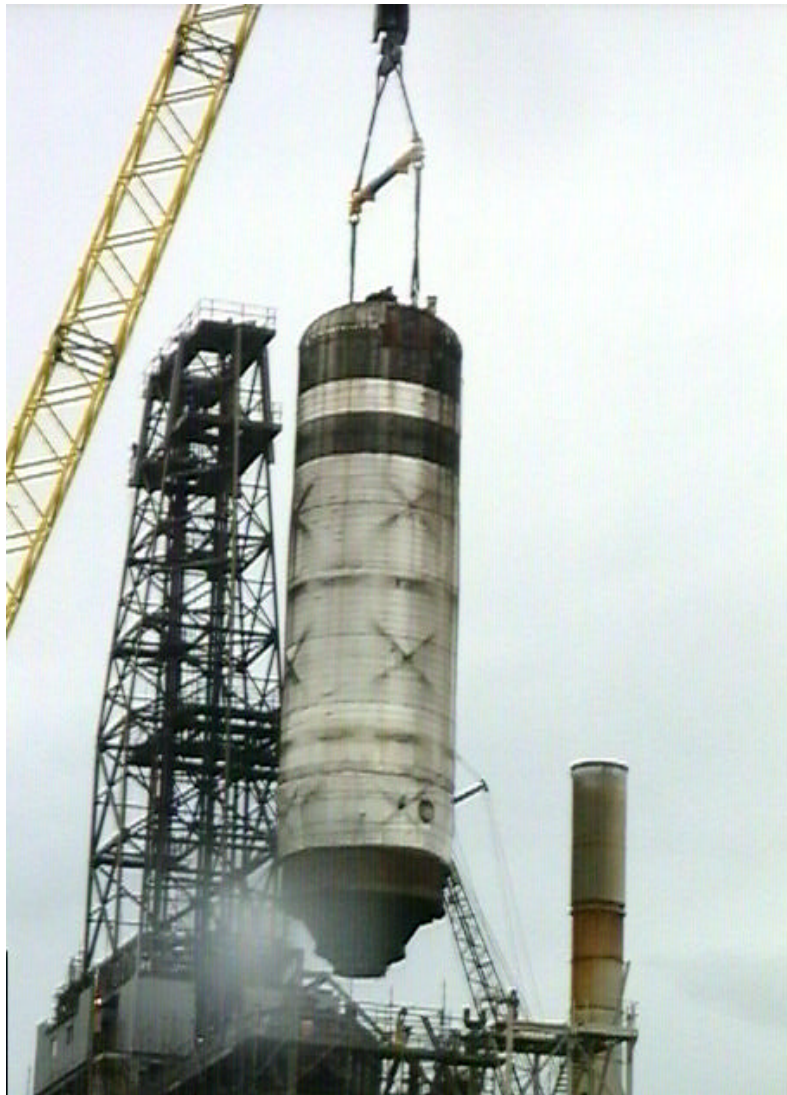
Figure 9: Removal of repaired coke drum which operated without problem until new drums were installed.
