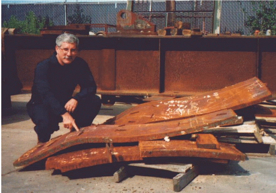
Figure 8: Dramatic examples of plate removed from drum demonstrate magnitude of bulge.
